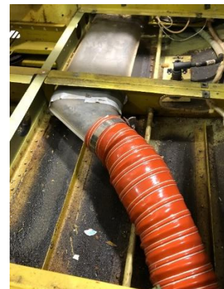
(right) New SCEET duct
