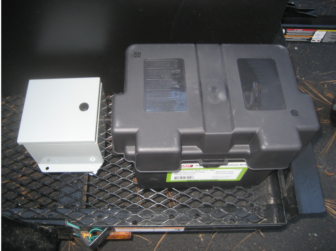
Battery Box And Control Box
